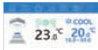
System Air Conditioner
