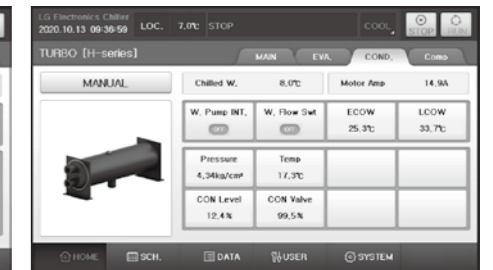
State of condenser
